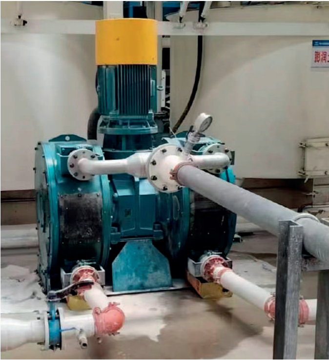
05 ▶ Strong acid and strong alkali pumping
